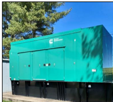
FULL BUILDING BACK-UP GENERATOR
