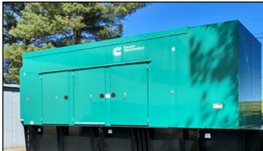
FULL BUILDING POWER BACK-UP GENERATOR
